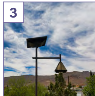
Solar Powered Street Lamps
